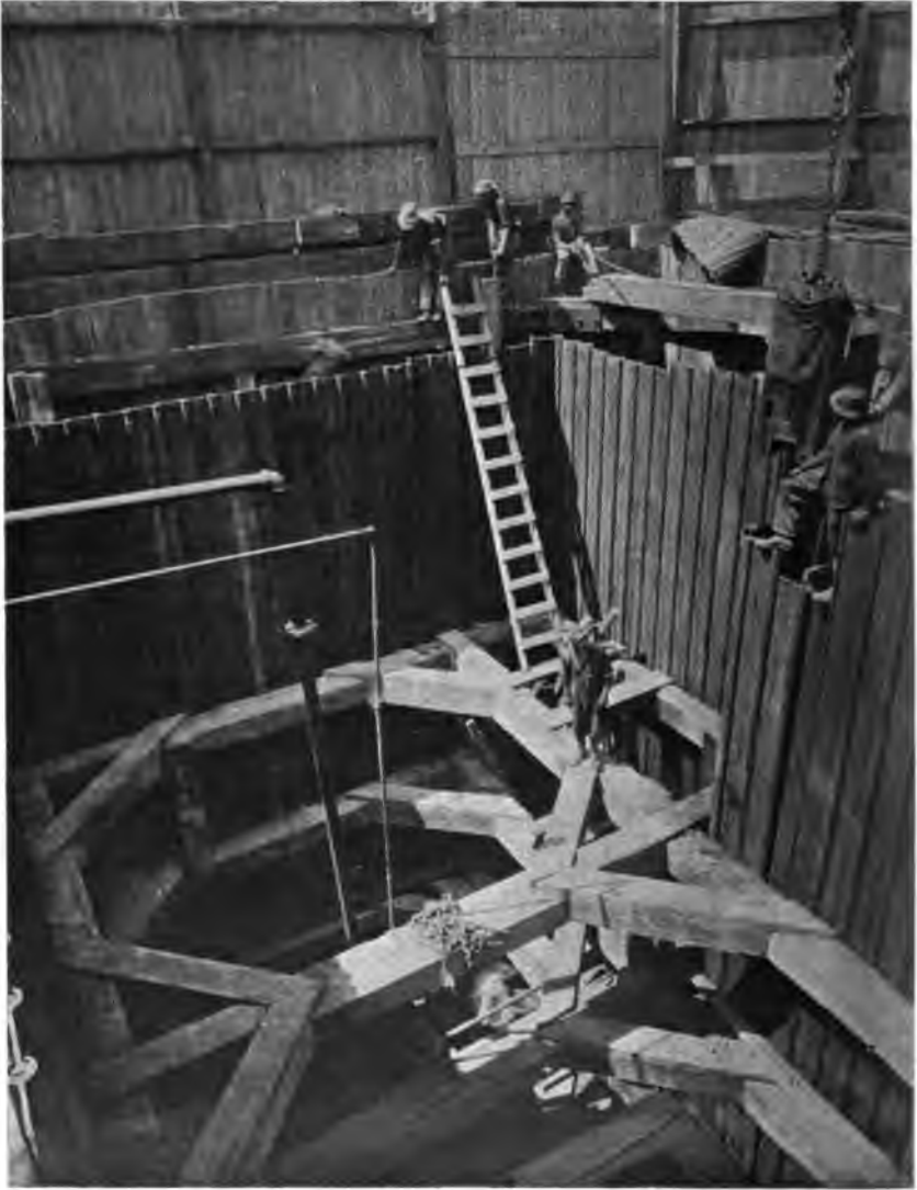
PLATE 218.—Contract 66. Shaft 18. Steel Sheet Piling Used to Reach Rock through Water-bearing Gravel. Piling driven by steam hammer.
